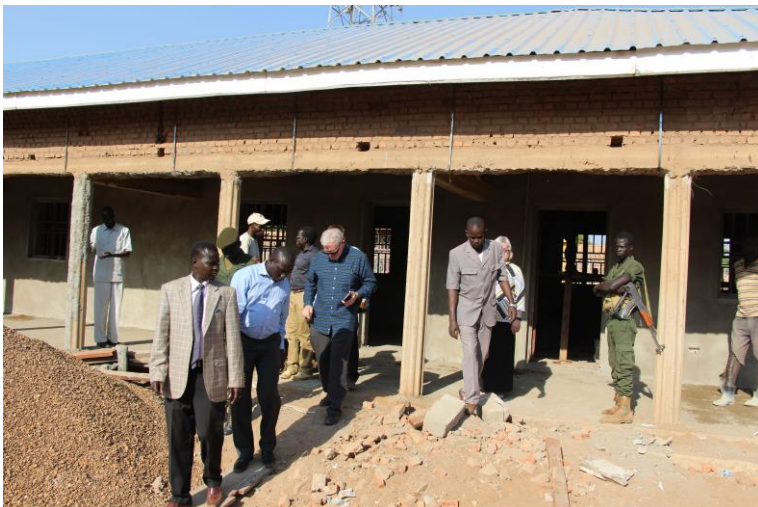
The SSAM team visiting the vocational school while it was under construction in January.
